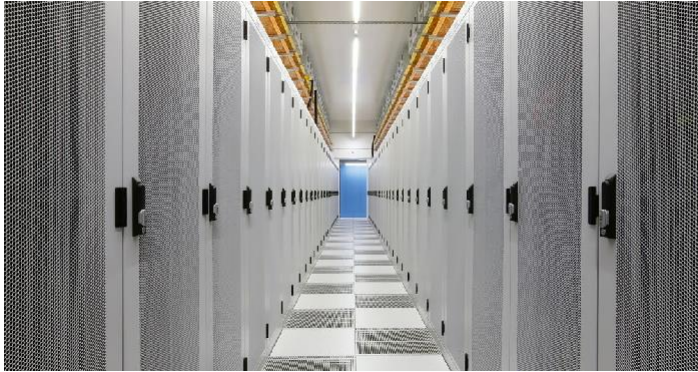
Xtream Server AM5 IBX data center interior
